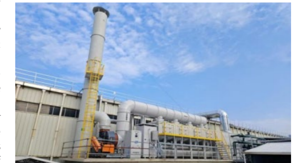
Newly Constructed Exhaust Gas Treatment Facilities
